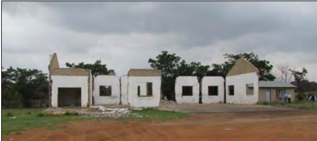
Figure 6-8: Dilapidated structure on Stand 88 built between 2005 and 2006 (Photograph by N Higgitt, 2013)
