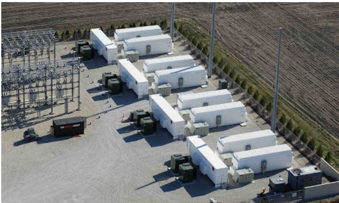
Plate 8-7: A stock image of a similar development with an on-site substation and BESS.
