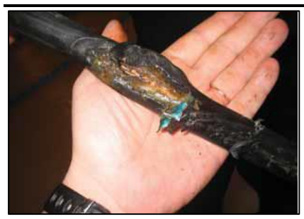
Figure 9.8 Photograph of cable damaged by a grapnel intended to retrieve fish traps from 1800 m depth.
