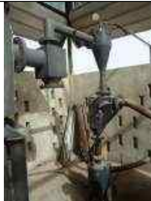
Square box and venturi scrubber
