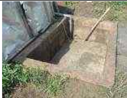
Biogas system pre-pit
