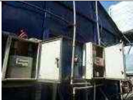
Digester gauges and gas meter (on the structure housing the digester bag)
