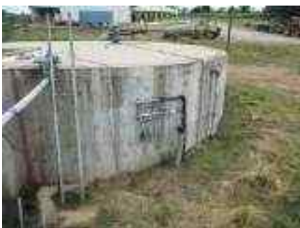
Digester 1 with inlet for heating pipes
