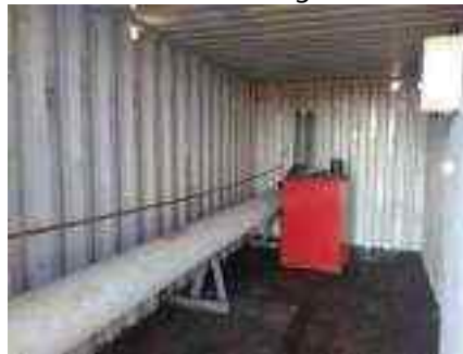
Heat exchanger powered by pellet boiler
