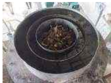
Feedstock on top of reactor
