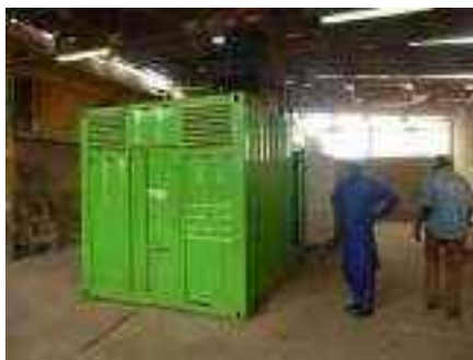
Engine container (heat exchanger on top) and desulphurisation unit
