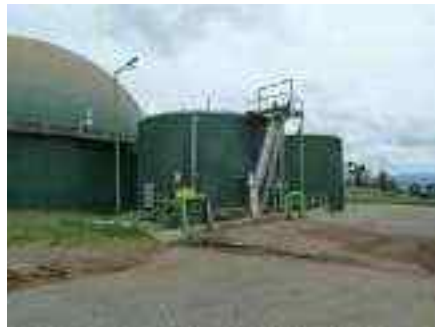
Feeder pump to tank 1
