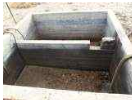
Waste water cement pond
