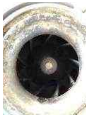
Damaged impeller blades
