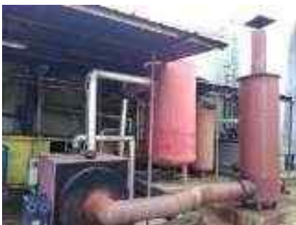
Diesel boiler with exhaust and water storage tanks
