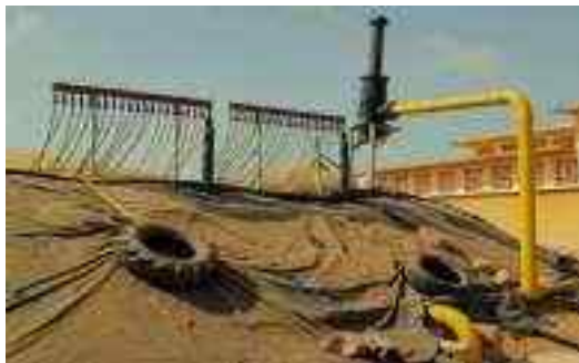
Heating pipes entering the digester
