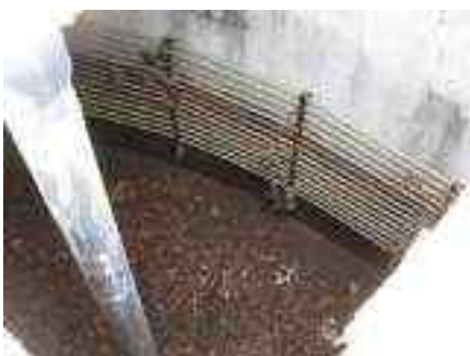
Empty (acidified) digester with internal heating pipes
