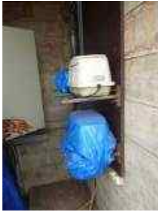
Air injection units
