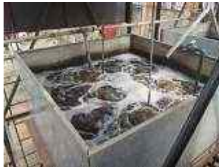
One of the aerobic reactor tanks
