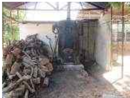
Boiler for heating pasteurising water (new system will replace)
