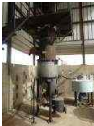
Gasifier feeder unit, hopper and reactor
