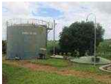
Hydrolysis tank (left) fed by collection tank (bottom right)
