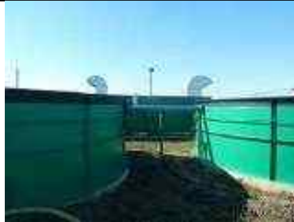
Second digester tank with interconnector (engine room behind)
