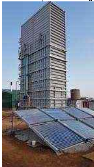
Picture taken in mid-July (reactors now upright; solar panels for pre-heating in foreground)
