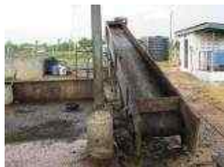
Feed conveyor for organic waste
