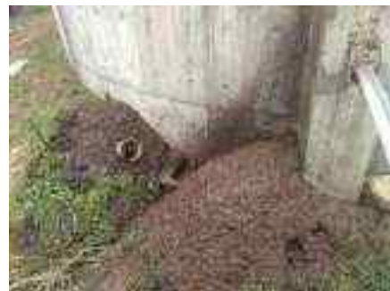
Solid slurry outside Digester 1
