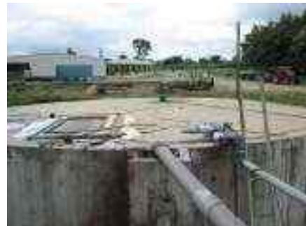
Digester 1 with overflow shaft
