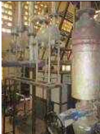
Cyclone and wet scrubbers
