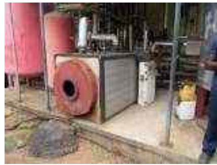
Dual-fuel diesel-biogas boiler
