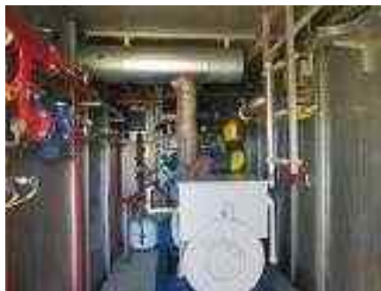
Deutz dual fuel CHP engine
