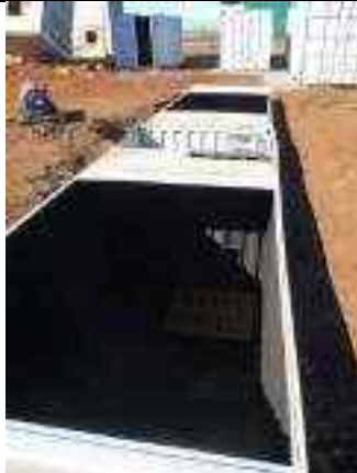
Two buffer tanks
