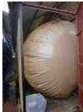
Biogas storage bag
