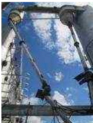
Cyclones & ash removal system
