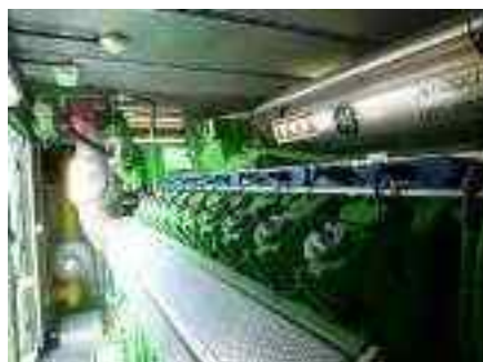
Jenbacher gas CHP engine
