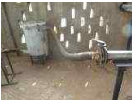
Emergency filter and manual gas injection handle
