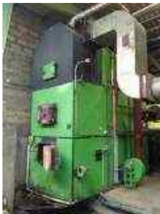
1,600 kWth biomass boiler in factory two
