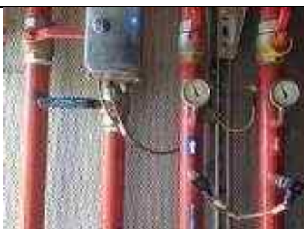
Heat transfer pipes from engine
