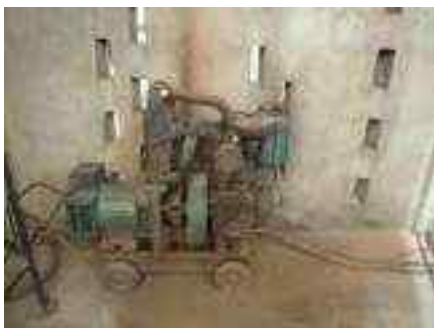
7.5kVA Start-up diesel generator
