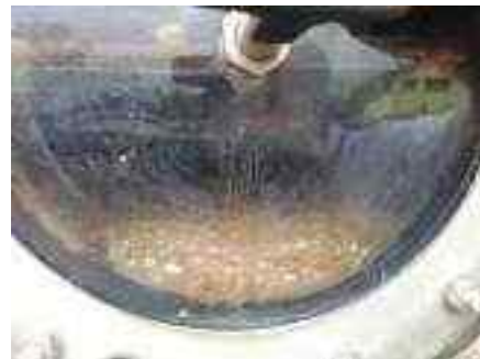
View through bulls eye of Digester 1
