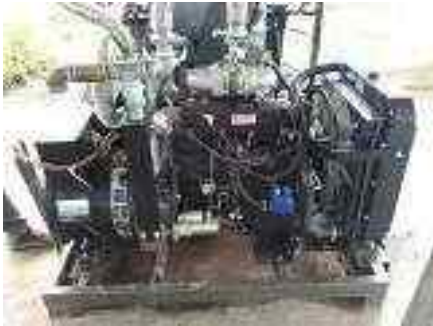
Engine and electricity generator
