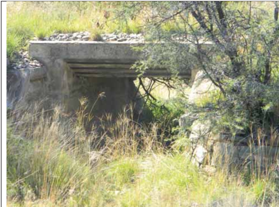
An example of a culvert that occurs in the Eastern Cape section
