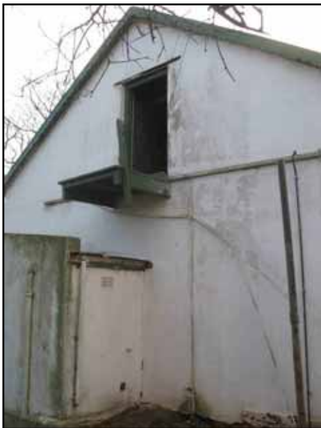
Figure 59: The southern end-gable with the solder staircase missing.
