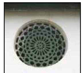
Figure 61: One of the many identical air vents positioned just below the roof.
