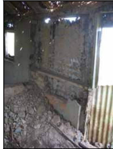
Figure 67: View of the inside of the ruined corrugated iron structure.
