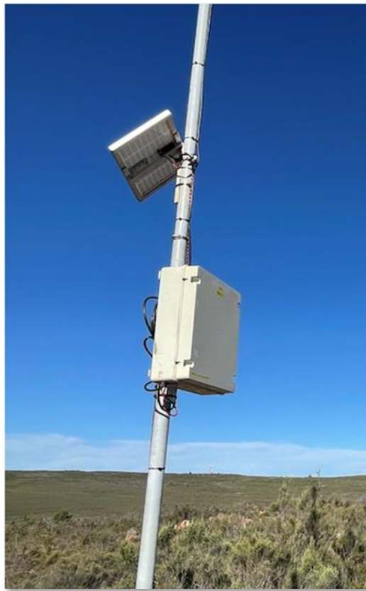
Figure 3: System on a 10 m mast at the proposed Hugo WEF.
