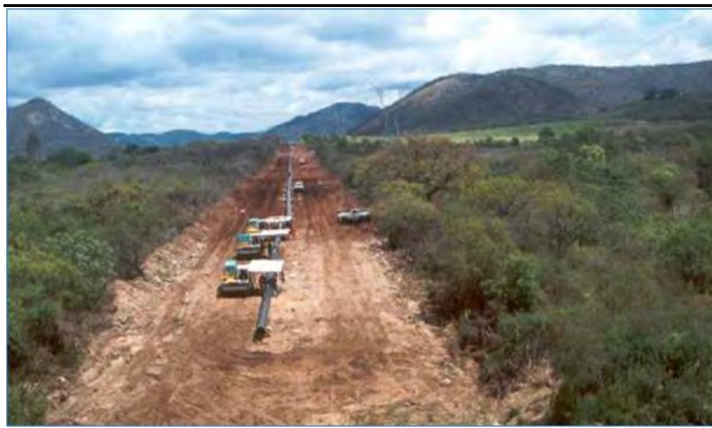
Figure 2.5 Example of the Construction of a Pipeline and Associated Right of Way
