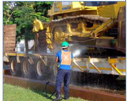
Cleaning of earth moving equipment brought into the loop line construction area for invasive plant prevention.
