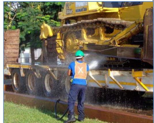
Cleaning of earth moving equipment brought into the loop line construction area for invasive plant prevention.
