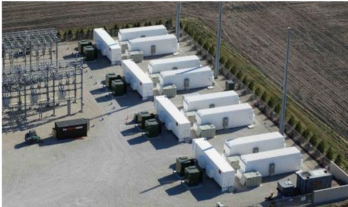
FIGURE 7-7: A STOCK IMAGE OF A SIMILAR DEVELOPMENT WITH AN ON-SITE SUBSTATION AND BESS.
