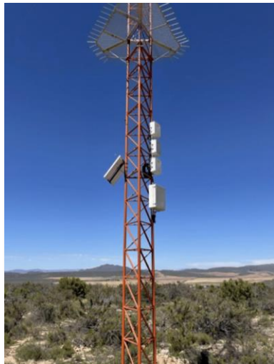
Figure 2: Systems deployed on the Met mast.
